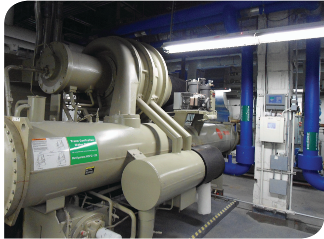
Chillers are optimized using the Trane Tracer Summit Chiller Plant Manager to reduce energy consumption.
